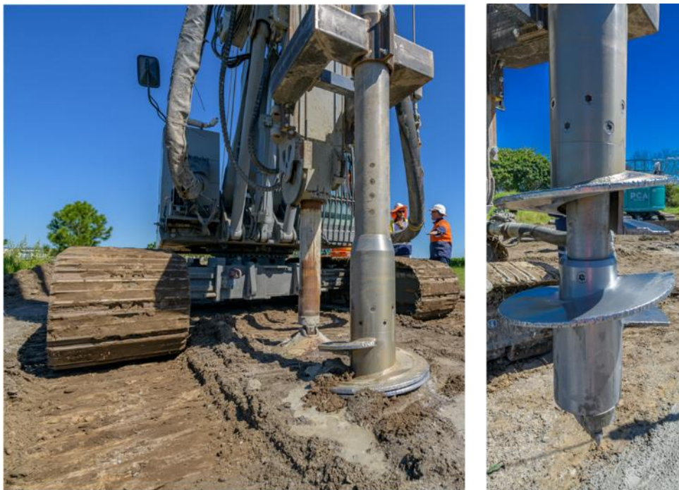
Figure 8: PAILE tool fitted to piling rig Comacchio CH450 with helical plates closed (left) and open (right).
